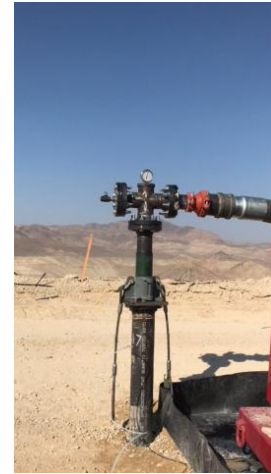
Figure 7. Typical high pressure injection well head
