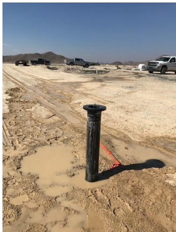
Figure 2. Typical completed injection well
